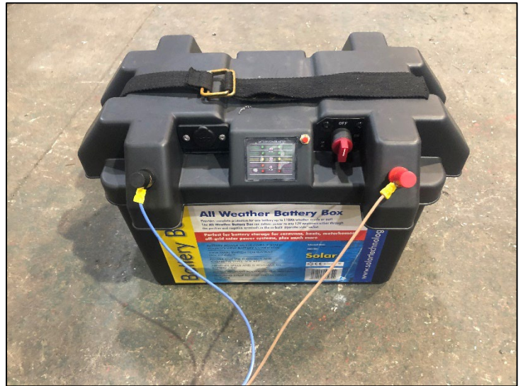
Fig 5 – Battery box – Power connection
